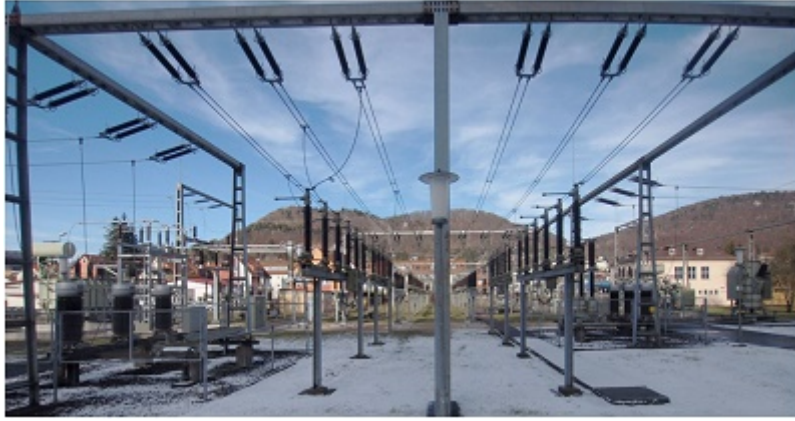
Figure 2 - High power cables connecting by busbars
